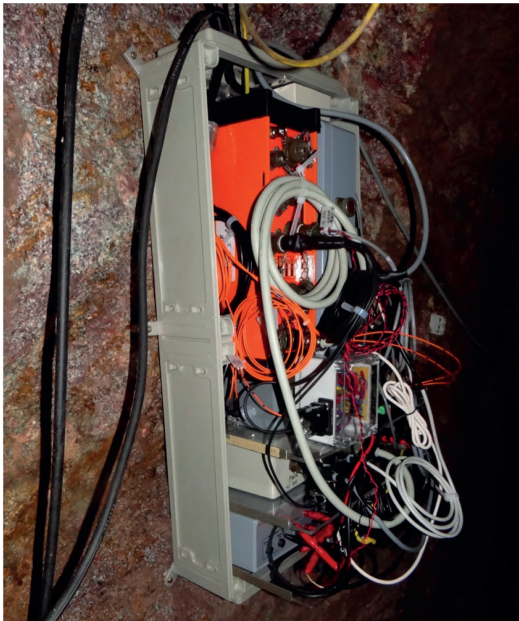
Figure 4.2: Electronics cabinet (with the cover removed) in the upper tunnel of the Anton mine. It houses the electronics units of the FGE and Overhauser magnetometers, the Q330 digitizer, the buffer amplifier, fiber optic media converters for LAN and PPS signals, a mini-PC, a Hygrometer and power supplies.
